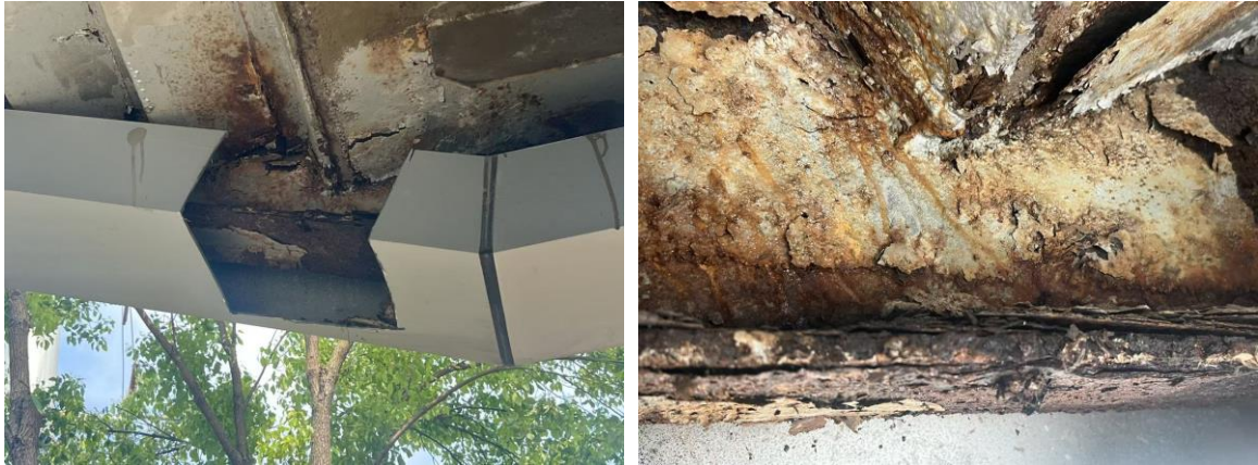
梯道主梁锈蚀
