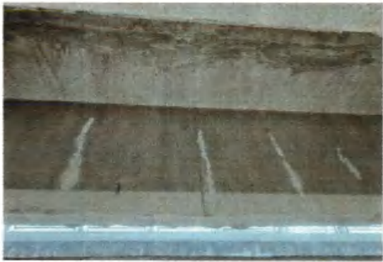
泛白吸附竖向裂缝
