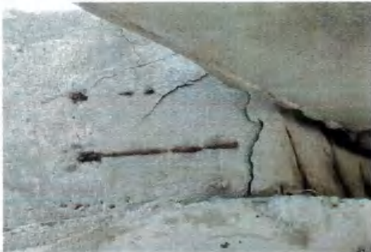
挡块锈胀露筋
