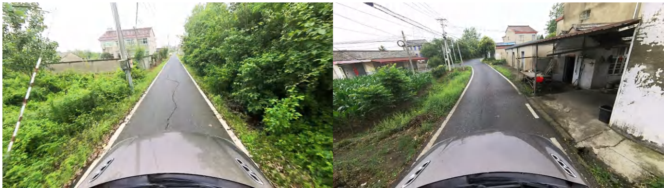
横向裂缝、纵向裂缝、修补
