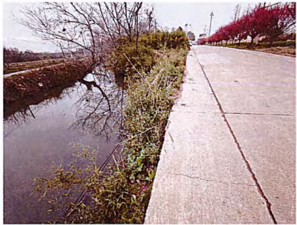
K0+270 处土路肩缺失
