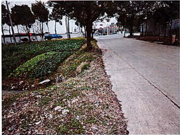
K0+043.5 涵洞土路肩缺失
