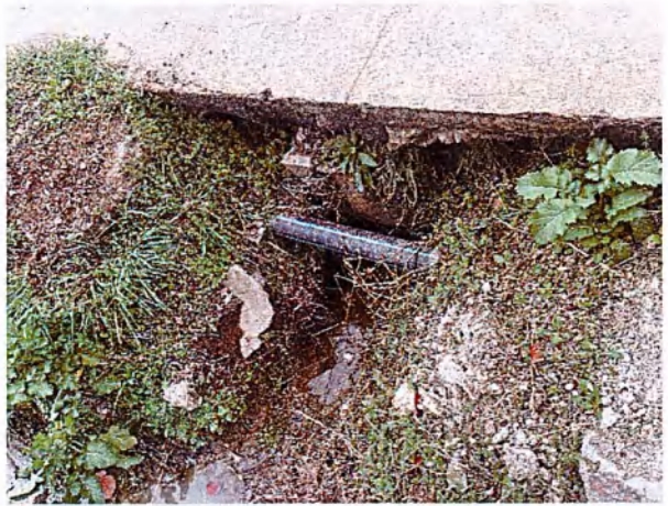
K0+507.029 处土路肩缺失
