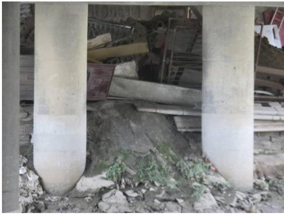
2-1#墩立柱小桩号面船撞破损
