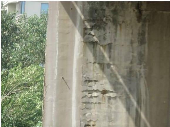
11#墩 1#盖梁小桩号面露筋锈蚀
