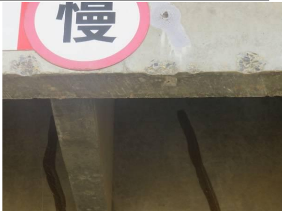
9-13#右腹板露筋锈蚀
