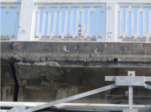
1#孔左侧人行护栏外侧面露筋锈蚀
