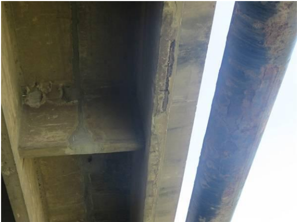
2-1#梁底板露筋锈蚀, 锈胀
