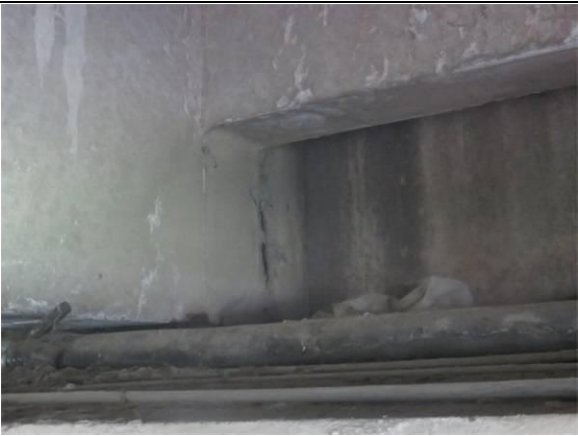
13-6#右腹板露筋锈蚀，破损
