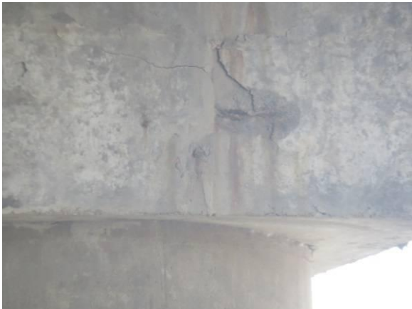
10#墩 1#盖梁小桩号面露筋锈蚀
