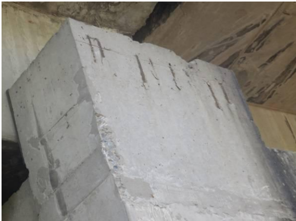
7#墩 1#盖梁右侧面露筋锈蚀
