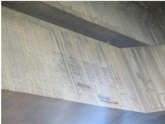
12#墩 1#盖梁小桩号面露筋锈蚀
