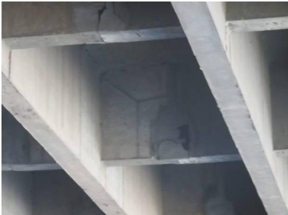
4-3-3#跨间横隔板连接钢板锈蚀
