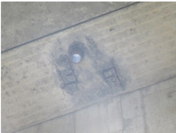
桥面板胀裂露筋锈蚀
