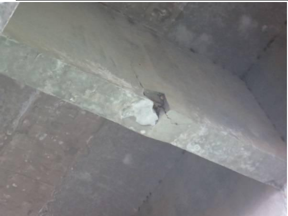
9-4-2#跨间横隔板大桩号面破损
