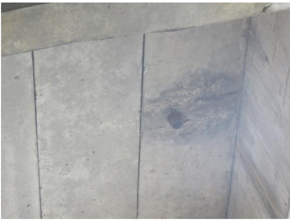
桥面板胀裂露筋锈蚀
