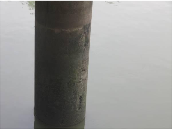
2-1#墩立柱大桩号面船撞破损
