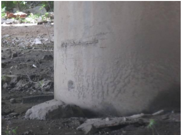
9-2#墩立柱小桩号面露筋锈蚀
