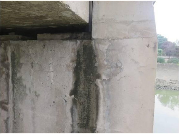
2#墩 1#盖梁大桩号面锈胀
