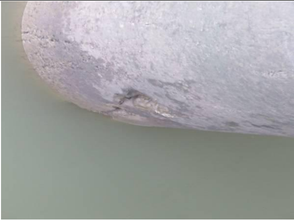
3-2#墩立柱小桩号面船撞破损
