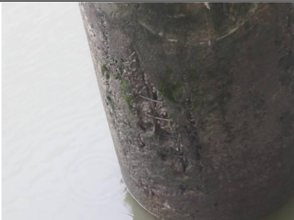
5-1#墩立柱大桩号面锈胀
