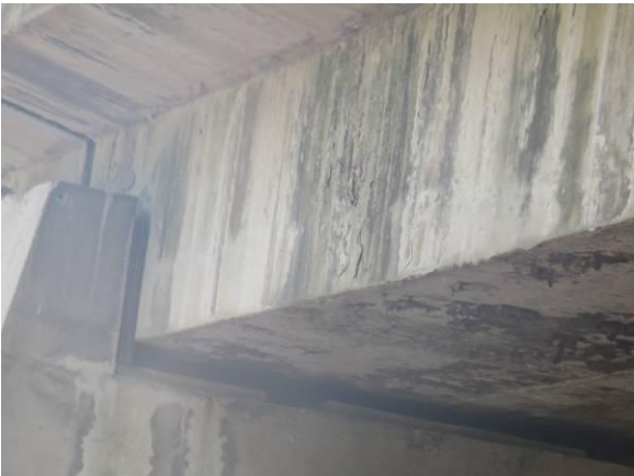
7-19#梁右腹板露筋锈蚀，锈胀
