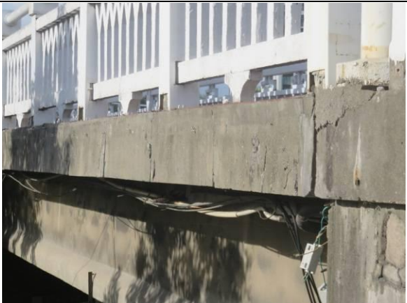
1#孔左侧人行护栏外侧面露筋锈蚀
