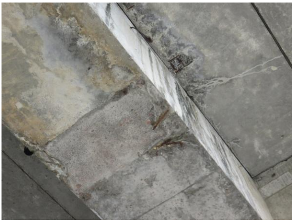
桥面板胀裂露筋锈蚀
