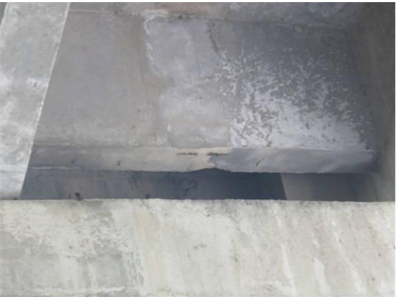
13-3-1#跨间横隔板露筋锈蚀
