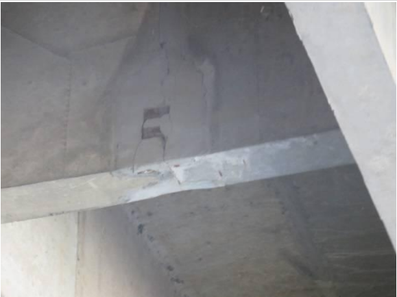
1-3-3#跨间横隔板连接钢板锈蚀
