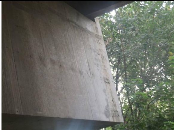
12#墩 1#盖梁大桩号面锈胀
