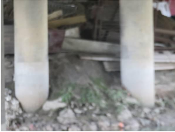
1-1#墩立柱大桩号面船撞破损
