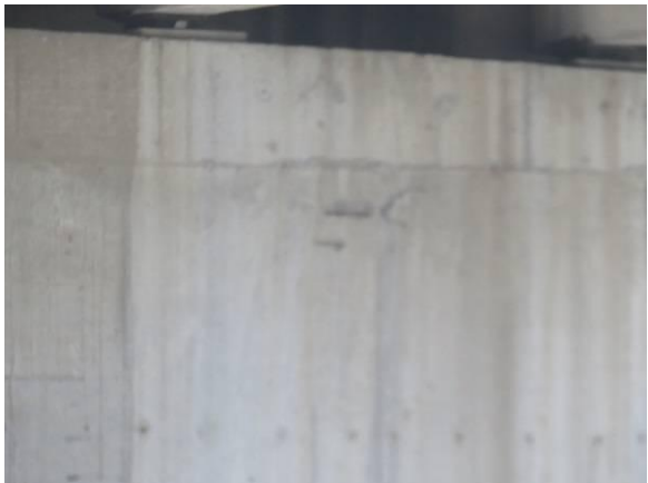
11#墩 1#盖梁小桩号面露筋锈蚀
