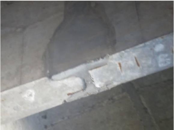
5-13-4#跨间横隔板锈胀，露筋锈蚀
