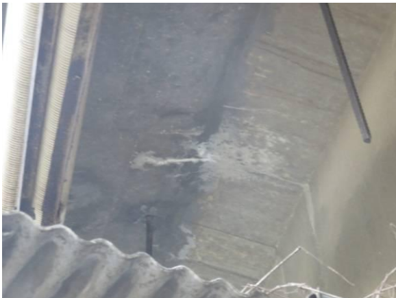
3-1#梁右翼板横向裂缝
