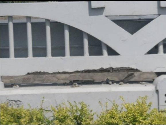
1#孔右侧人行护栏露筋锈蚀
