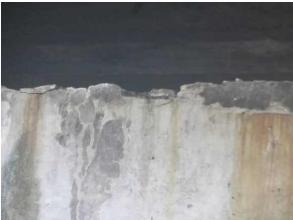
8#墩 1#盖梁大桩号面锈胀
