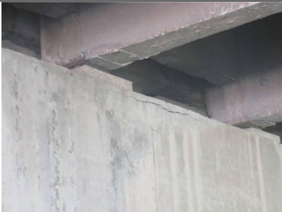
7#墩 1#盖梁大桩号面锈胀
