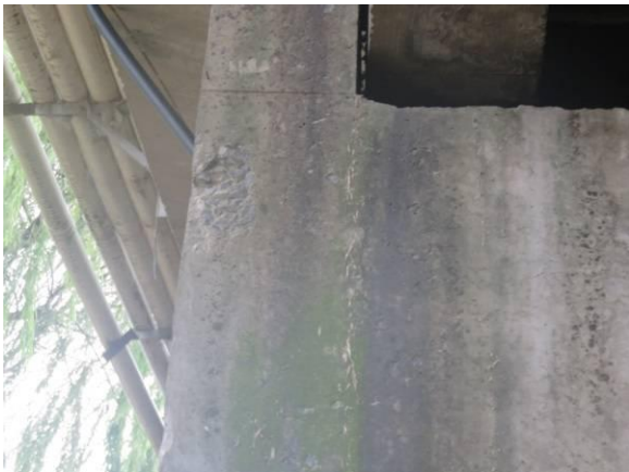
8#墩 1#盖梁大桩号面破损
