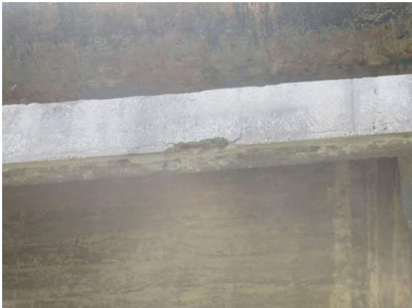
2-1#梁底板露筋锈蚀, 锈胀
