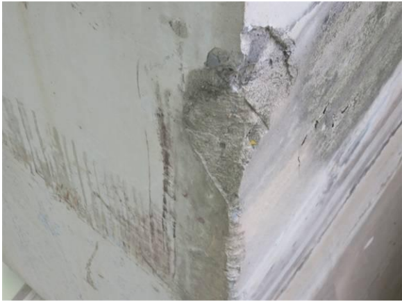
2#墩 1#盖梁小桩号面露筋锈蚀
