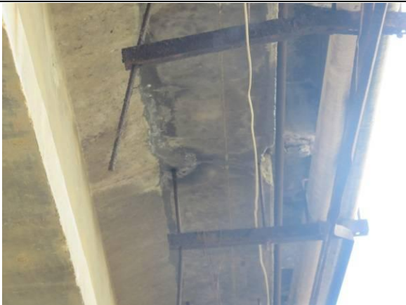
1-1#梁右翼板渗水侵蚀
