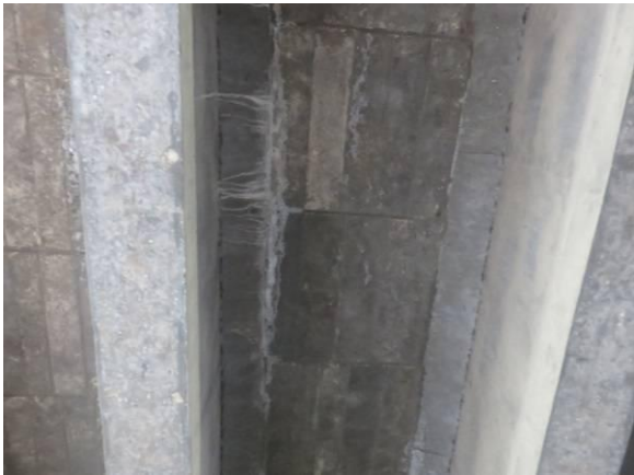
3-3#桥面板纵向裂缝
