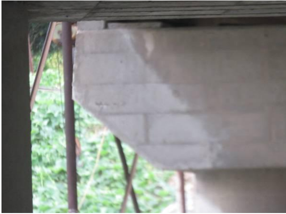
1#墩 1#盖梁大桩号面露筋锈蚀
