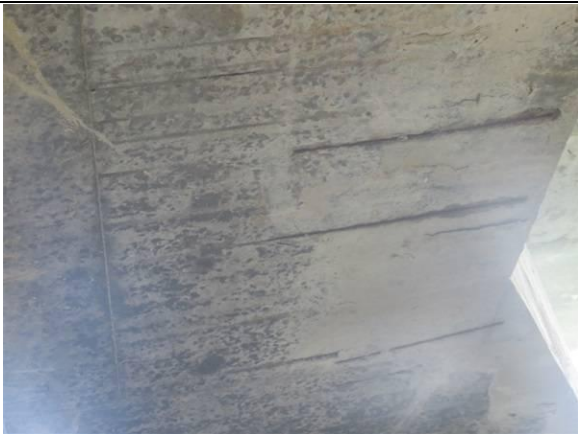
12#墩 1#盖梁底面露筋锈蚀
