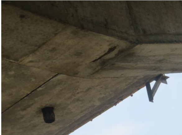
12-2#横梁底面，距左边缘 3.0m 胀裂露筋锈蚀
