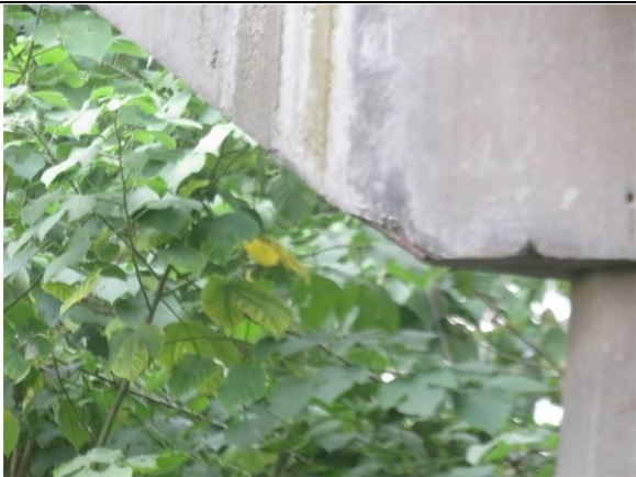
9#墩 1#盖梁小桩号面露筋锈蚀，破损
