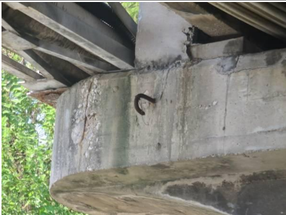
1#墩盖梁大桩号面露筋锈蚀，锈胀
