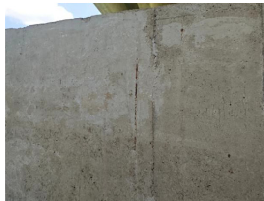
58-2#系梁锈胀露筋
