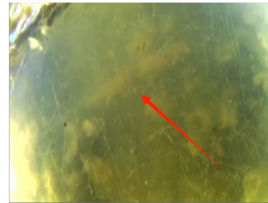
57-1#桩砼破损、露筋
