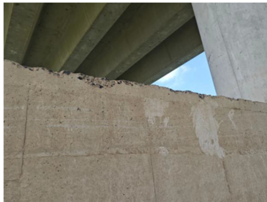
64-2#系梁锈胀露筋
