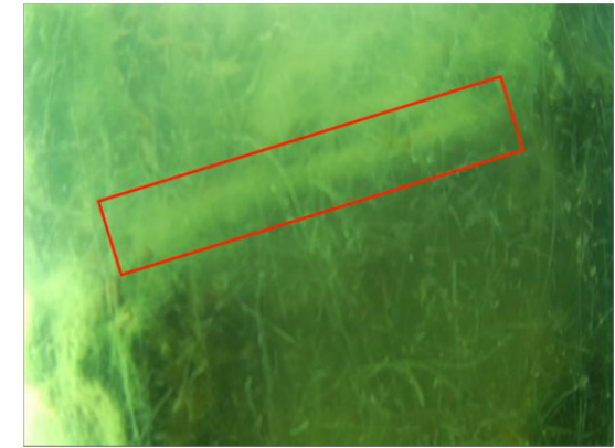
41-2#桩砼破损、露筋
