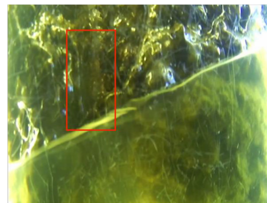
59-1#桩砼破损、露筋
