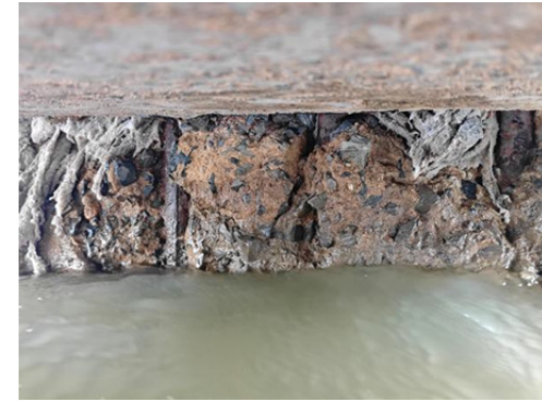
42-1#桩砼破损、露筋
