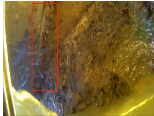
62-2#桩砼破损、露筋
