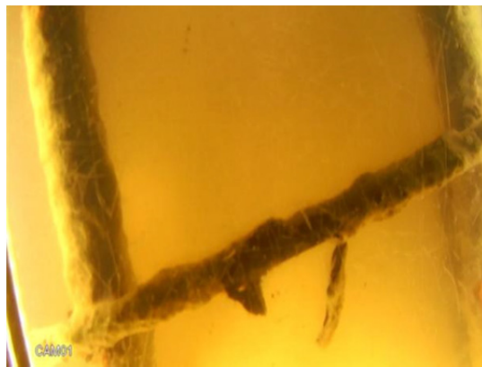
59-2#桩砼破损、露筋
