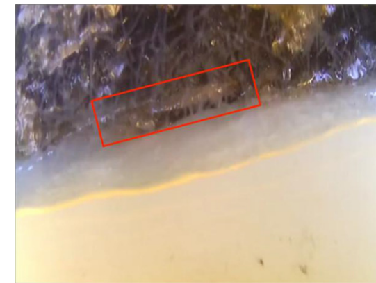
53-2#桩砼破损、露筋
