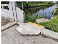
护栏构件断裂
